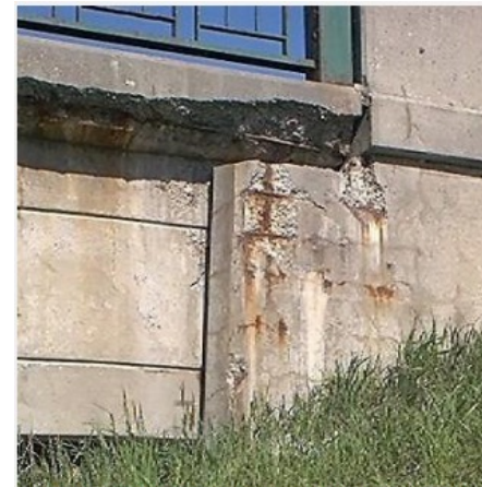
Low concrete cover and no protective coatings gave the rebars no protection from atmospheric acid attack
